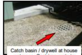
Catch basin / drywell at house entrance. Cast iron grate is flush to ground surface
