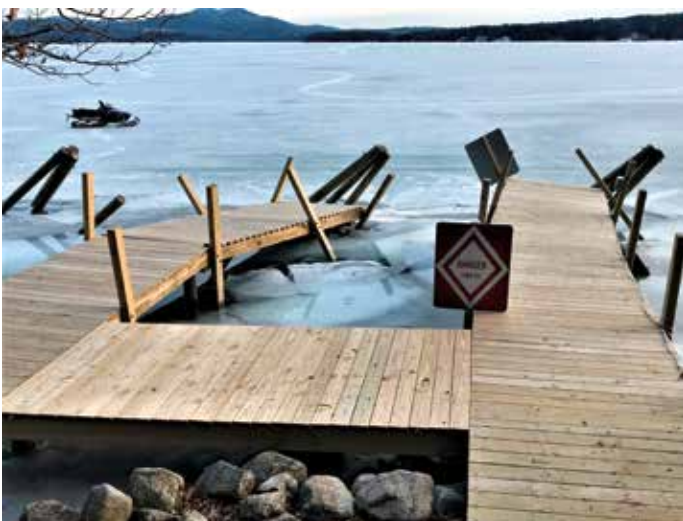
Ice damage caused by improper de-icing techniques. (Photo Credit: Watermark Marine Systems, LLC)
